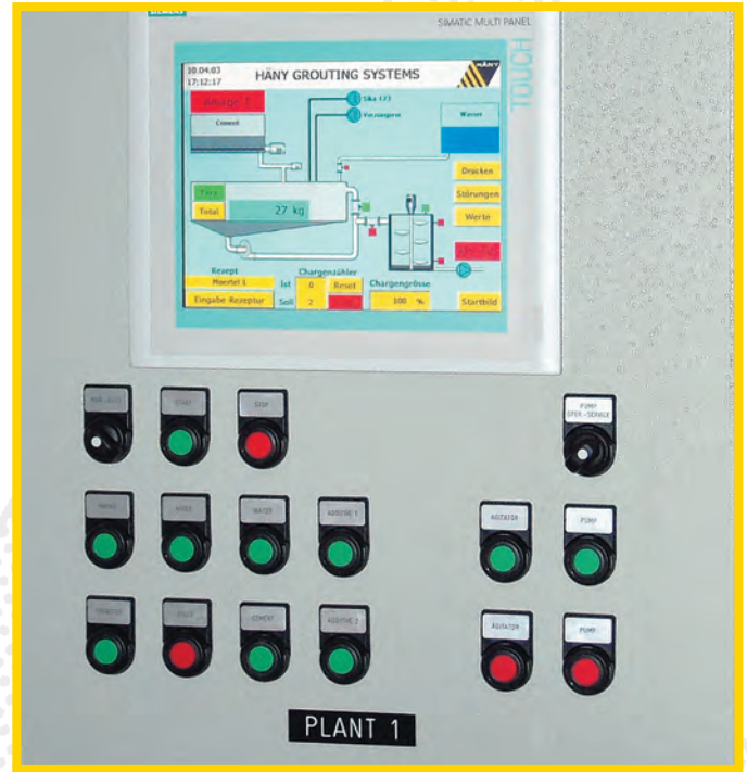
Electric control with touch screen panel.
