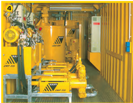
3) Automated mixing plant MCI 2000/726 with ZMP 726 high performance pump for the transport of grout suspension (W/C ratio 0.7) over a distance of 3,750 m. Boston.
