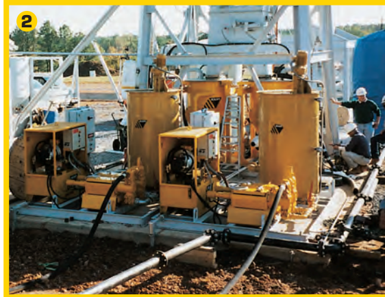
1) Channel Tunnel Rail Link-CTRL Contract 240: PLC controlled backfill plant with ZMP 712 and ZMP 725 grout pumps. London.
