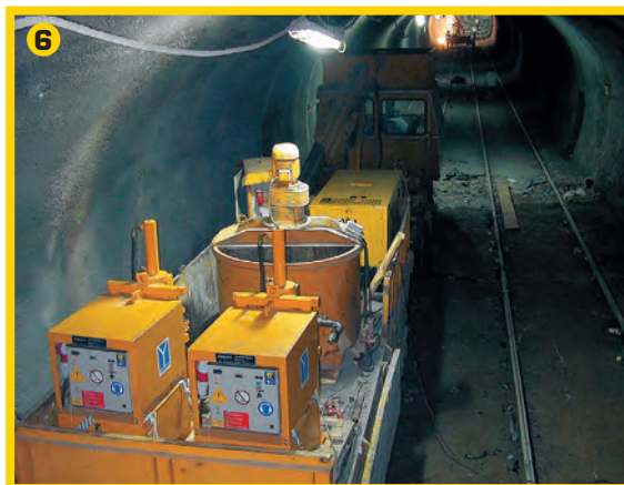
5) Grout plant with automated weigh-batching and four grout pumps for general grouting work. Bratislava.
